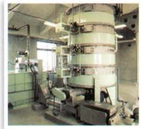
Sludge Treatment Equipment
